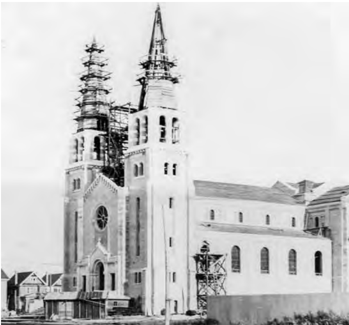
The Holy Rosary Cathedral, located at the southeast corner of 13th Avenue and Garnet Street, under-construction in 1913. (City of Regina Archives CORA-F-0797)
