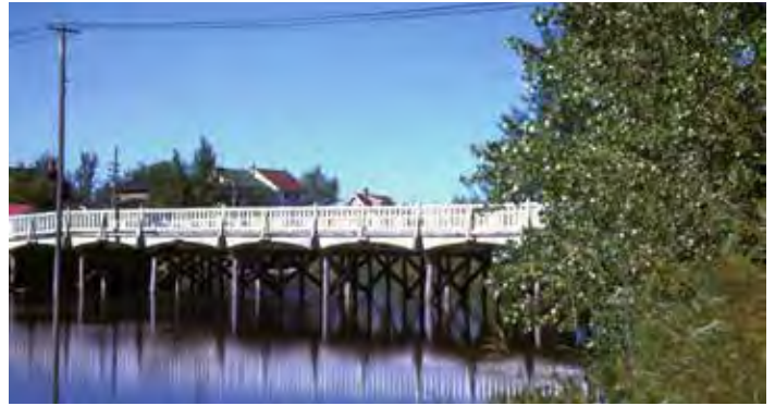
The wooden Retallack Street traffic bridge over Wascana Creek in 1946. Baker, Everett (Saskatchewan History & Folklore Society SHFS 6077-X4)
